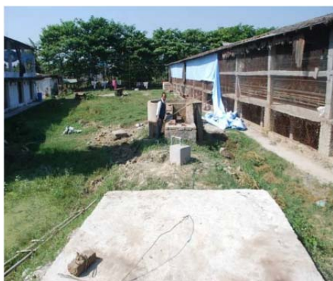
Biogas Digester on Poultry Farm
